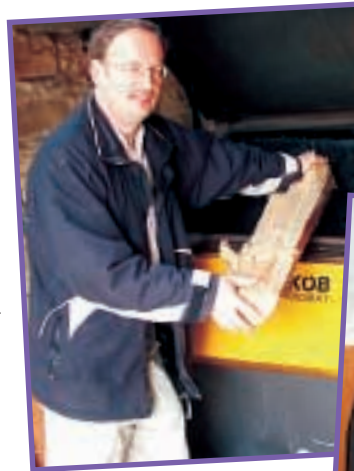
Erwin refuels the wood burning boiler with some of Botton's home-grown timber.
